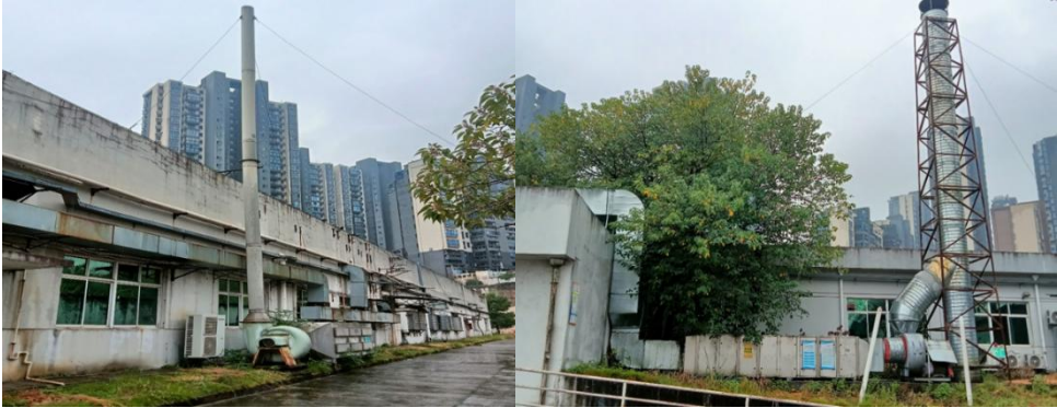
Waste gas treatment facilities (part)
