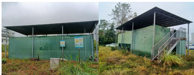
Wastewater treatment equipment
